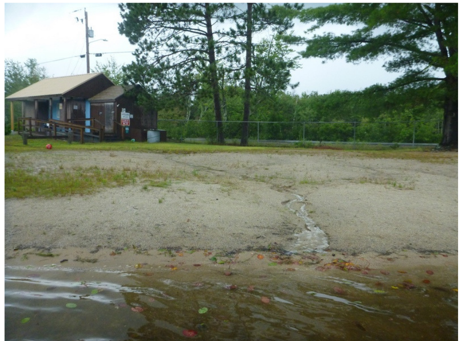
Figure 5.13. Drainage from Gregg Lake Road and the beach parking lot across the beach into Gregg Lake.
