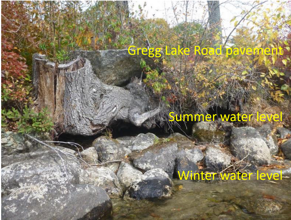
Figure 5.6. Undercut of bank close to Gregg Lake Road at summer water level. Photo taken with water at winter level, with both flash boards removed and water just flowing over dam.
