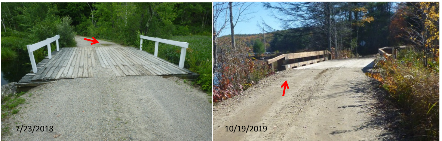
Figure 5.4. Left: Erosion Site 06 viewed from the south, showing severe erosion of Craig Road causeway and bridge shoulders, high water level on west (left) side of bridge due to beaver dam underneath and location of filled sinkhole, which had opened up in 2018 (arrow). Right: Site 06 viewed from the north, after bridge replacement. Sinkhole location still visible (arrow).
