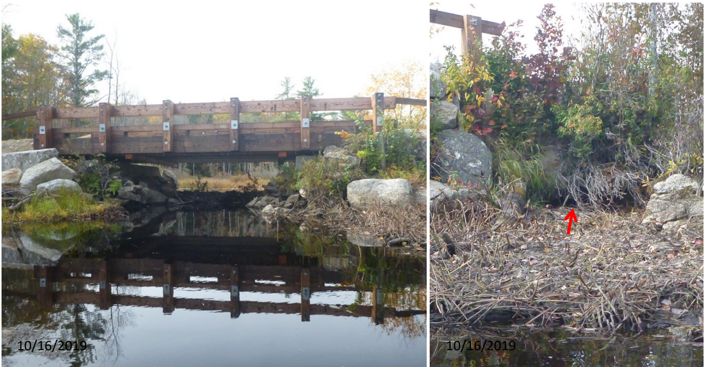
Figure 5.5. Beaver dam under new Craig Road bridge (left), with downstream water level lowered by approximately 16 inches after removal of flash boards at Gregg Lake dam. Bank erosion and probable sinkhole drainage site (arrow) at high water level made visible by low water level.
