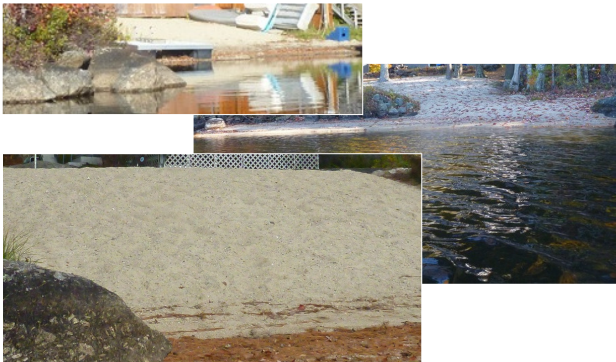
Figure 6.1. Severe erosion sites where sand has been dumped recently to create beaches on Gregg Lake.
