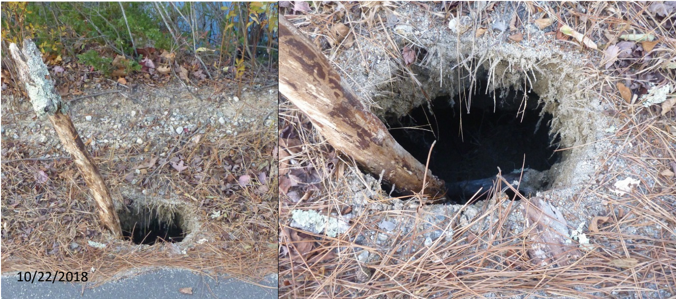
Figure 5.11. Sinkhole approximately 3 feet in diameter and 3 feet deep, with water visible at the bottom, found on Gregg Lake Road causeway Fall 2018.
