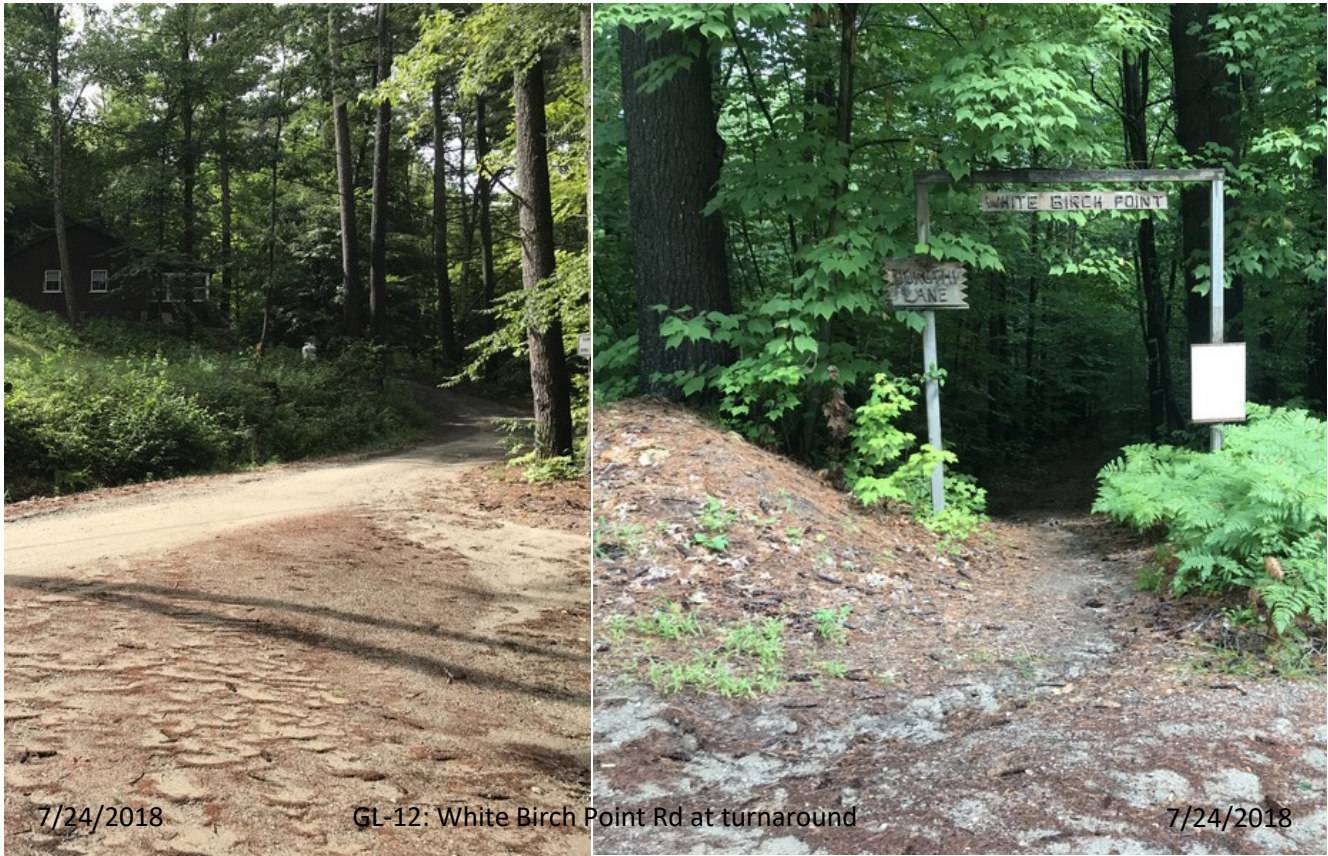
Figure 5.2. Erosion Site 12, where stormwater runoff from the upper section of White Birch Point Road flows across the turnout (left) and enters the steep access road to the White Birch Point private beach (right) or an adjacent private driveway.
