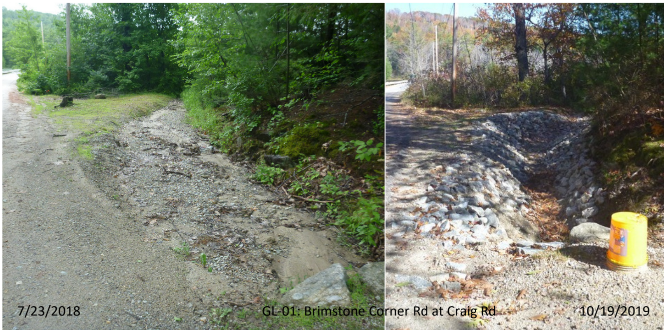
Figure 5.1. Erosion Site 01 at the intersection of Brimstone Corner Road, Craig Road and Gregg Lake Road, where stormwater runoff carries sediment down a steep section of Brimstone Corner Road and deposits it directly into Gregg Lake. Photos taken at the outlet of the culvert under Harbor Road looking towards Gregg Lake before (left) and after (right) installation of uphill turnouts and diversion dams, lining ditches, crowning, stabilizing road shoulders and installing a catch basin.
