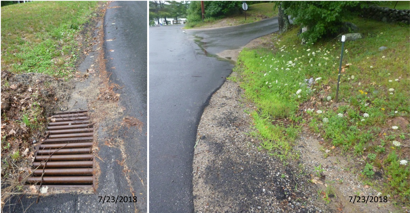
Figure 5.3. Erosion Site 09, where stormwater flows down Holt Hill Road, crosses Gregg Lake Road and washes across private beaches to enter Gregg Lake. A recently-constructed catch basin directs some of the flow under the road (left). Suggested area for installing a catch basin for remaining flow directed across Holt Hill Road, with storm drain in place (right). Ditch maintenance will be increased as needed to retain sediment.
